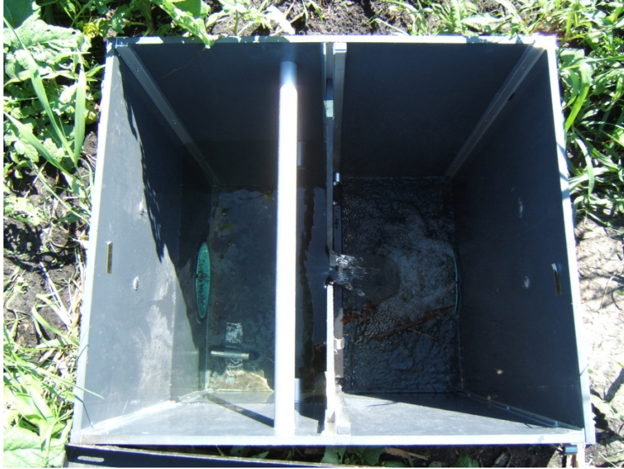
Figure 14. Bachand Tile Drainage Water Control Structure
